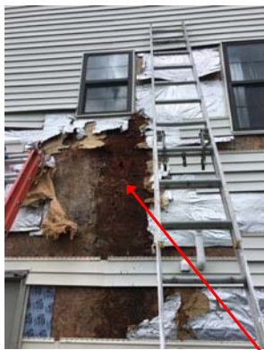
Major rot due to leaking window and lack of rough opening flashing.
