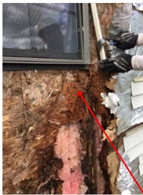
Resulting sheathing and framing rot due to lack of flashing at window.
