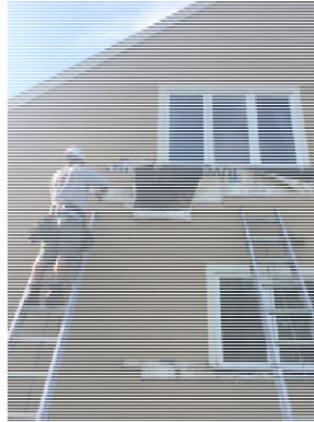
Verified envelope failure.
