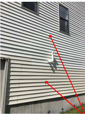
Previous repair performed. Note: different shades of vinyl siding.
