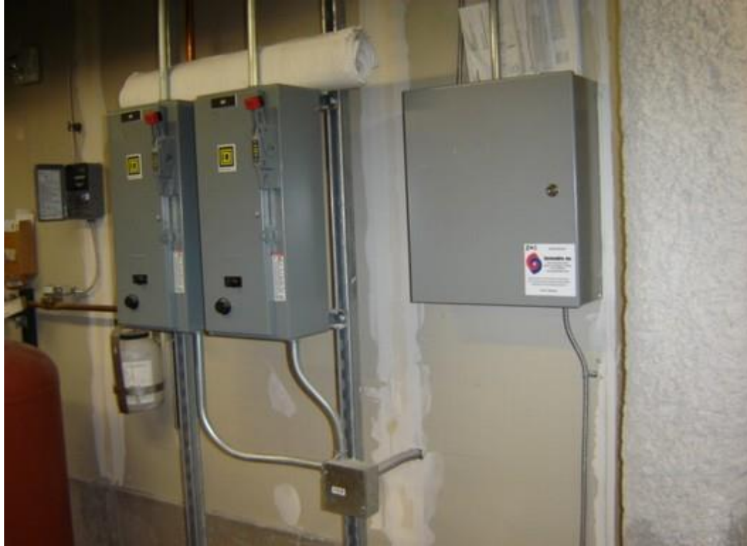
Cooling tower pump controls
