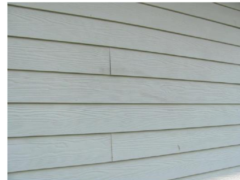
Discolored finish at Unit 200
