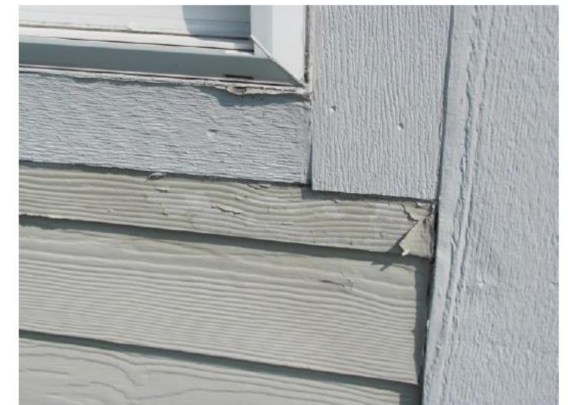
Peeling paint finish at Unit 300
