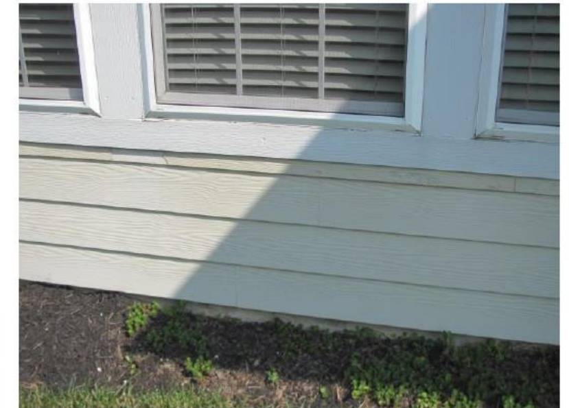
Sealant deterioration and peeling finish at fiber cement, Unit 100
